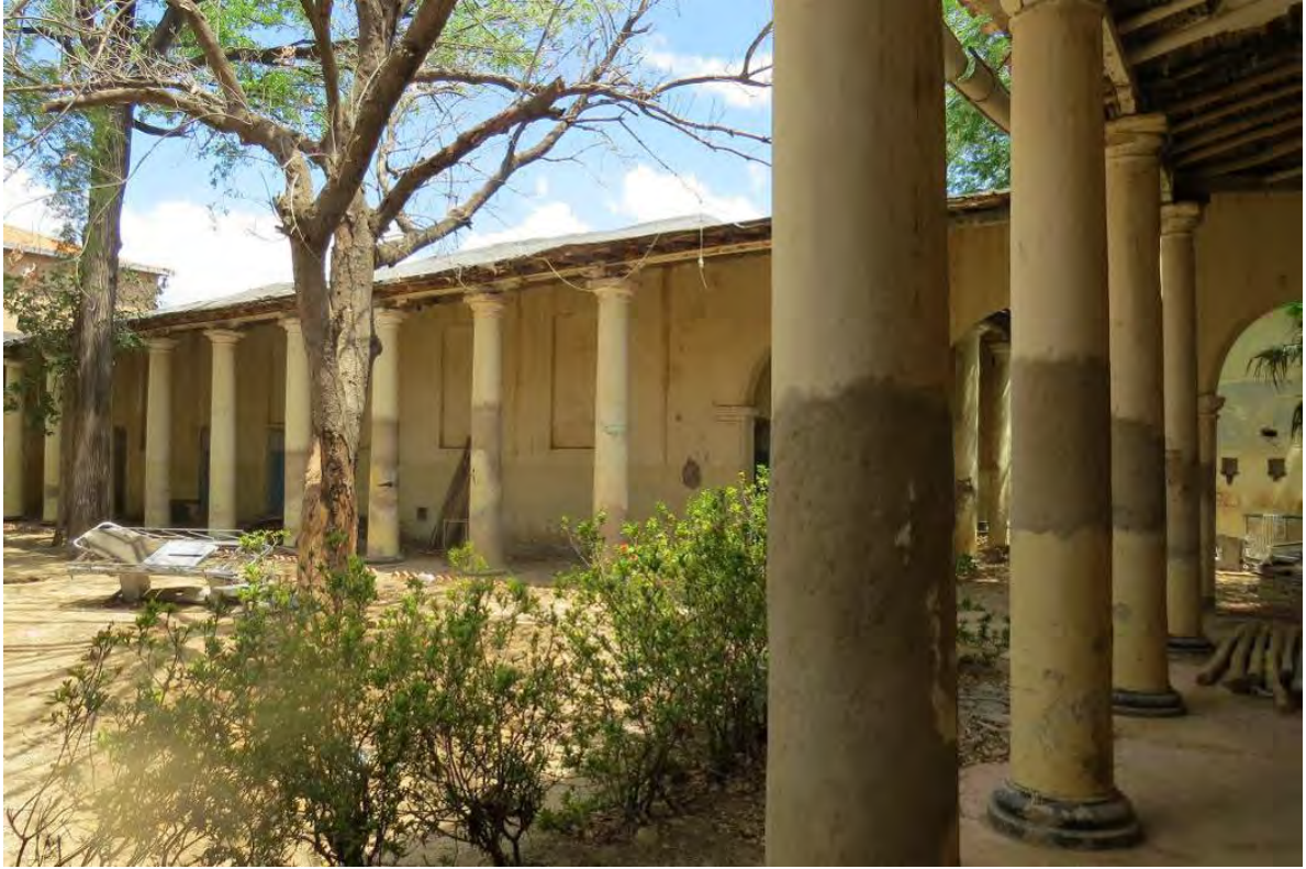
Photographs 20-21. Actual works of restauration in the Old Hospital using traditional techniques
