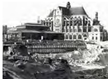
Demolition of historic buildings at the centuries-old Parisian marketplace, Les Halles. Photo: © J. Deneux, 1974.
