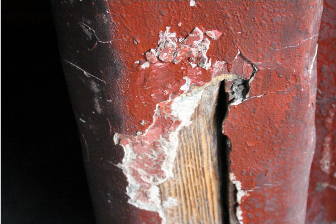
Damaged lime plaster over wooden members and columns. Such damages are noted at few specific locations
