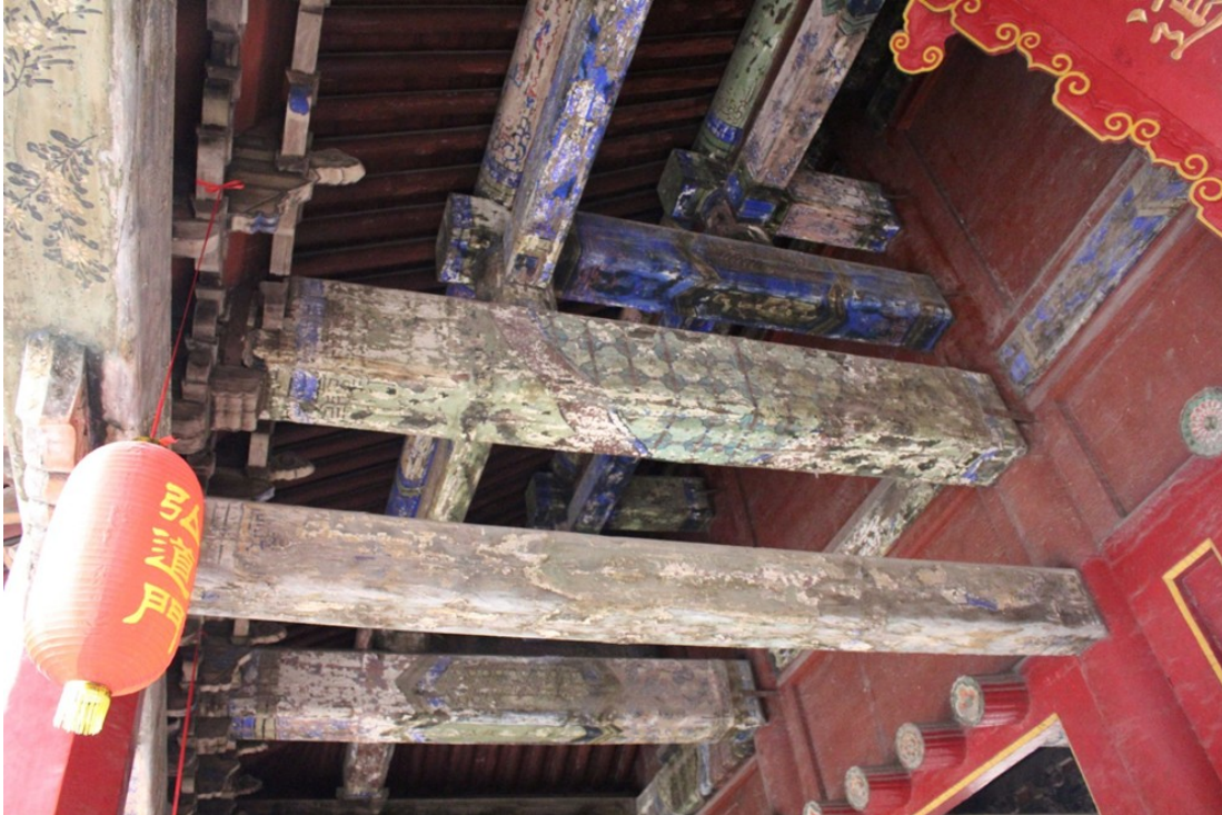
Art work on the wooden members needs urgent attention for conservation
