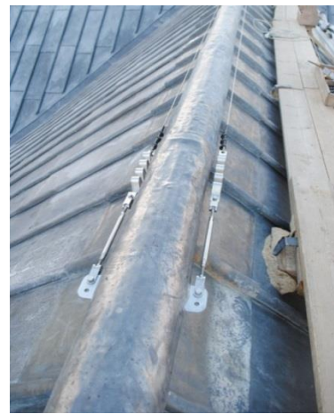
Figure 13: Installed life line at the roof
