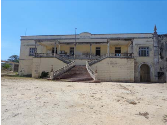
Fig. 8 Mozambique Island court of justice in progressive degradation
