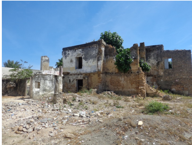
Fig. 10 Private ruin in high degradation situation
