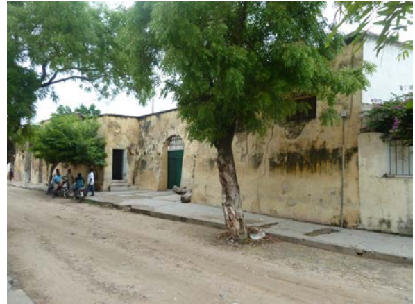
Fig. 9 District jail in progressive state of degradation
