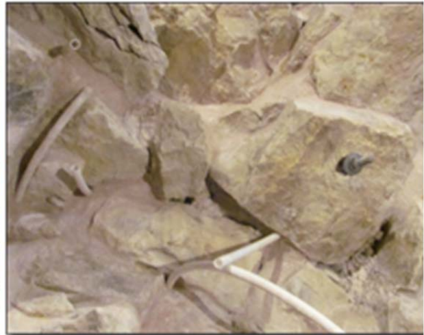
Fig. 2 – plastic pipe not injected
