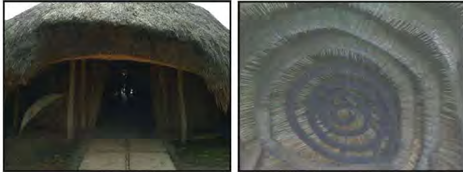
Fig 2: images showing the condition of the Bujjabukula
