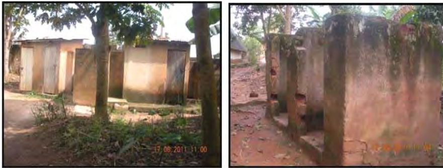
Fig. 12a pit latrines (L) and bath areas(R) for workers behind the katalama structure; the state of the buildings does not supports safe livelihood, and therefore the need for demolition or restructuring.
