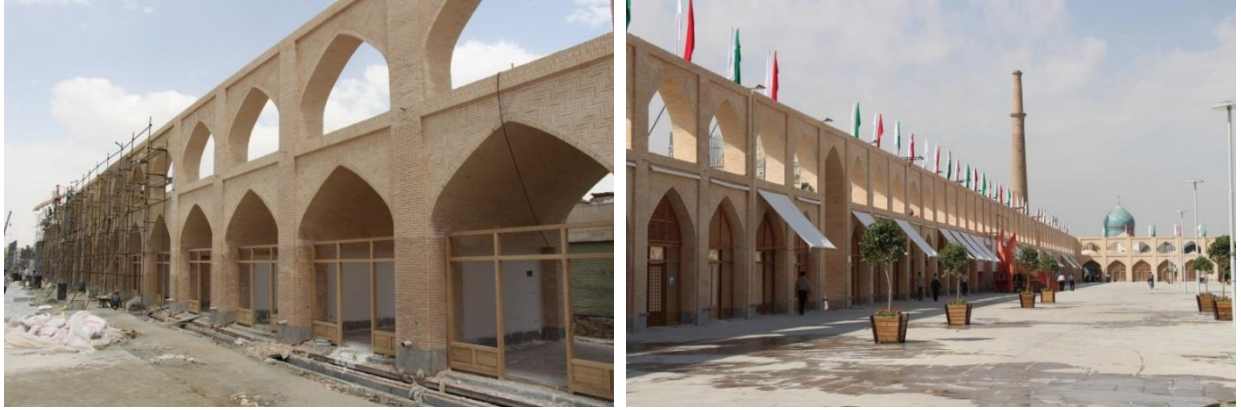
Figure 10. Eastern side of the Southern Section- Ongoing rehabilitation process (left), Outcome of rehabilitation plan (right)
