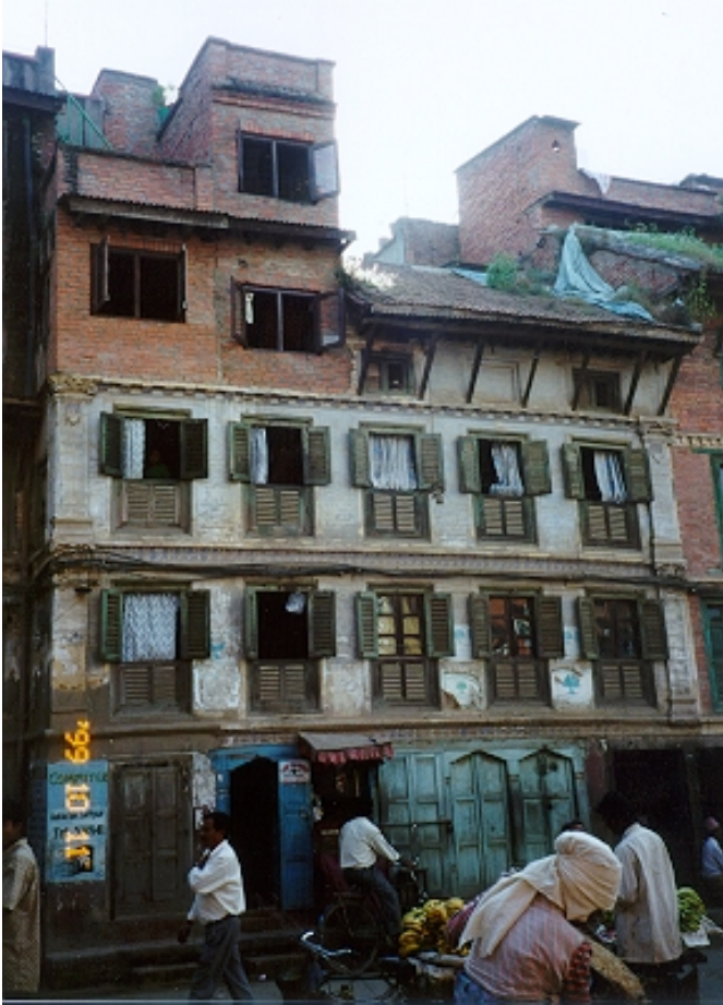
(Above) Two new floors were added in March 1999 after partial demolition of the original sloped roof.
