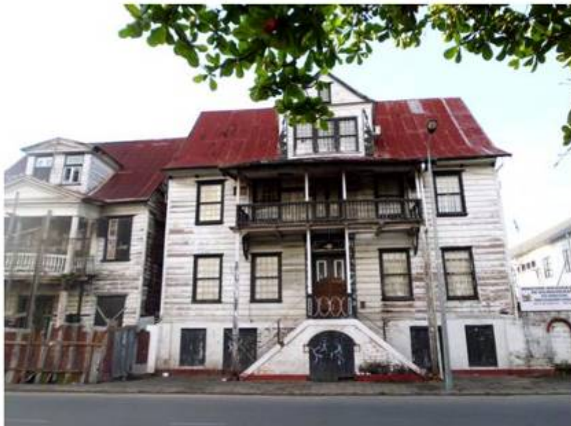
An outstanding but deteriorated house on the Waterfront
