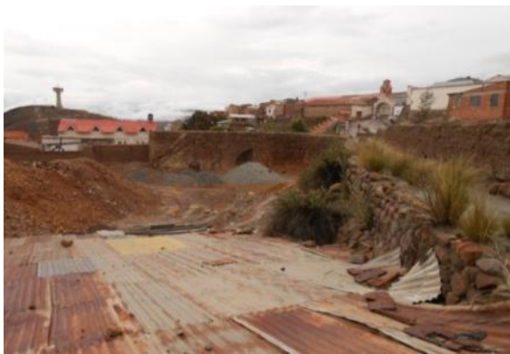
The uncontrolled inclusion of new architecture without consideration of the traditional building types of Potosí can affect the authenticity and integrity of the site.
