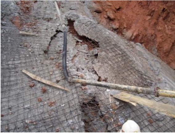
Fracture of the filling structure caused by the recent collapses in the Cerro Rico caused by the extraction of mineral and heavy rainfall.
