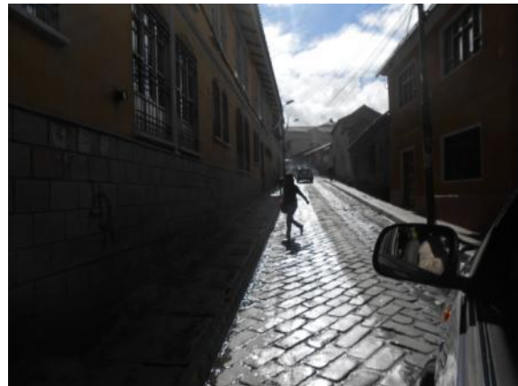
Carved stone pavement partially covered with asphalt.
