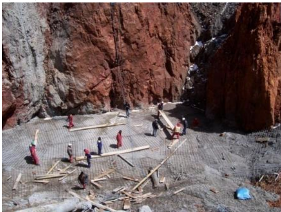
Beginning of the dome of the filler bracket. Photo Empresa Q & Q.
