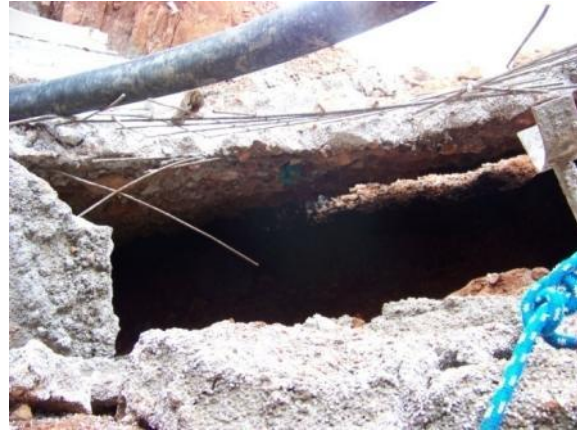
Collapse of the structure of filling.
