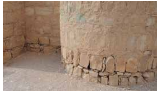
3.13. Hollow masonry at the bottom of the external walls, caused by flood (before conservation)
