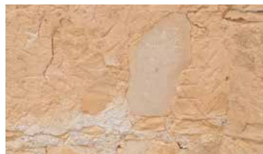
3.12. Plaster on the rear facade of the monument, with regular herringbone-patterned signs
