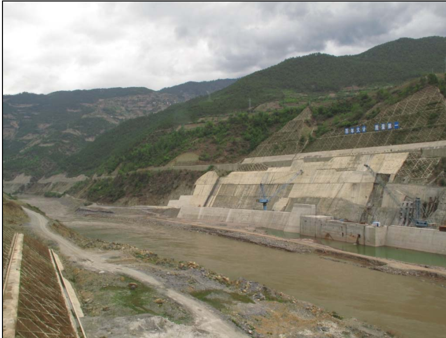
Photograph 1. Construction at the Lidi proposed dam site on the Lan Cang River (Upper Mekong River). Photo taken on 22 April 2013.
