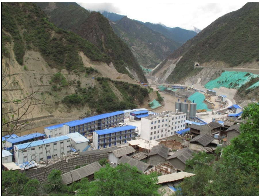
Photograph 2. Construction at the Wulongnong proposed dam site on the Lan Cang River (Upper Mekong River). Photo taken on 22 April 2013.
