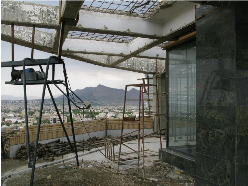
Figure 15. Demolition works of 11th floor at Jahan Nama building. State at May 7
