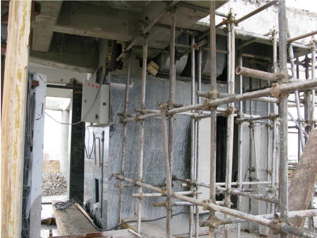
Figure 16. Demolition works of 11th floor at Jahan Nama building. State at May 7
