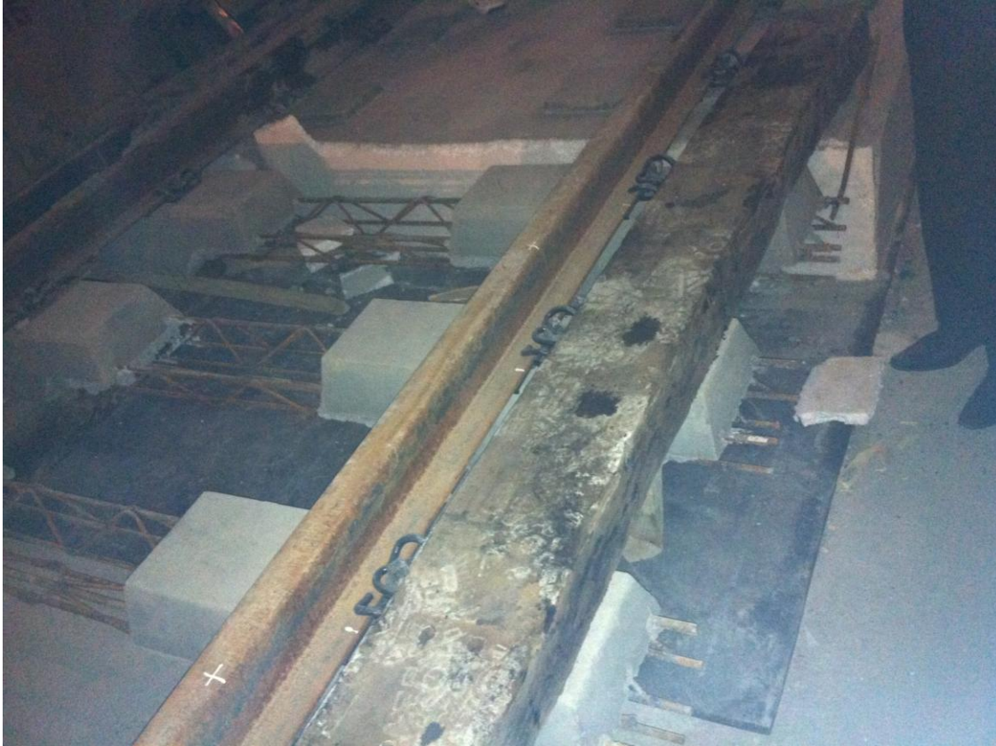
Figure 11. Full surface support Floating Slab Track under construction at Phase 1, Metro Line 1.
