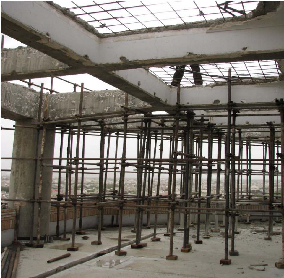
Figure 13. Demolition works of 11th floor at Jahan Nama building. State at January 17 (picture provided by ICHHTO)
