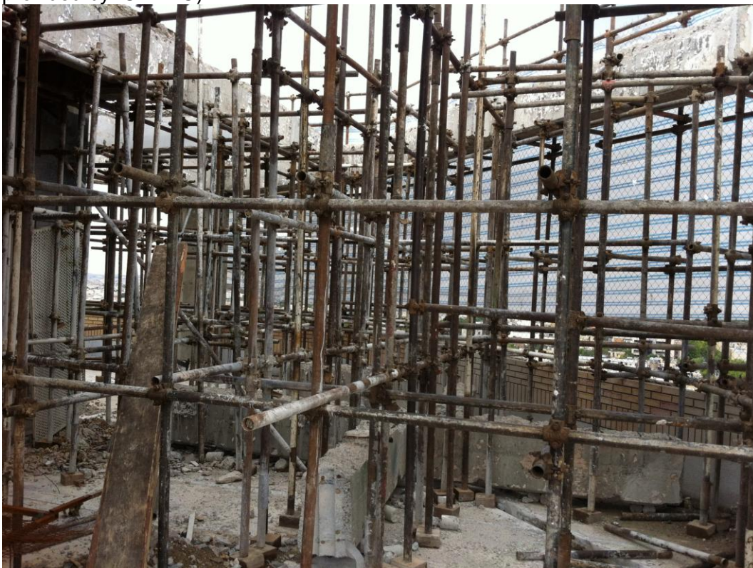
Figure 14. Demolition works of 11th floor at Jahan Nama building. State at May 7
