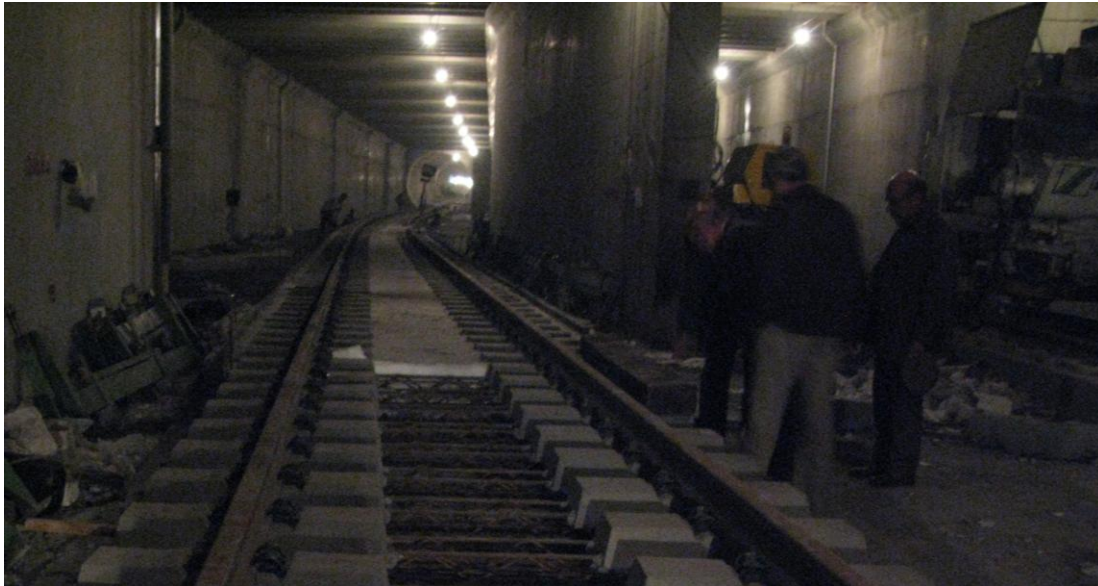
Figure 7. Transition of cut and cover section (Metro line 1, phase 1) to two Tunnels section (phase 2)
