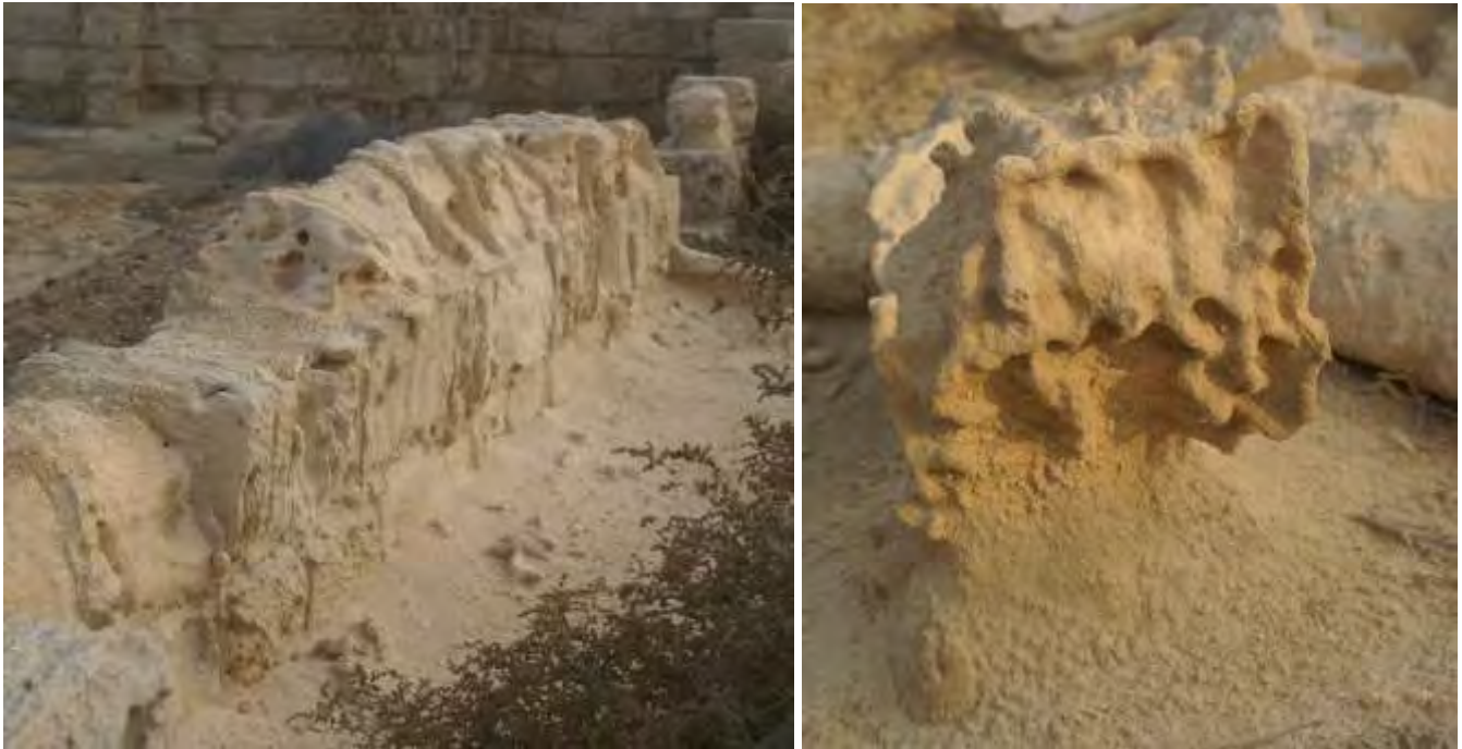
Figure 12. Extremely aggressive soluble salt deterioration of building blocks
