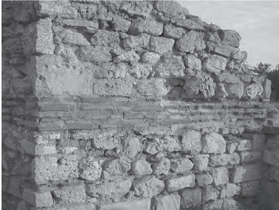
Figure 5. Example of wall elevation demonstrating several of the survey criteria. The wall has not been capped, but is reasonably stable and would therefore receive an average score for 'condition of wall top'. Accelerated loss from brick courses was highlighted by the staff of the NPTC as a particular problem on the site. The untreated area on the right would therefore result in a very low 'condition of wall elevation' score for the grid square in which this section of wall falls. The section of brick course to the left has been treated and is thus not an immediate problem and would not therefore result in a low score for 'condition of wall elevation' as, although inappropriate, the treatment is protecting the original material it is covering. It would, however, be noted as 'presence of previous treatment' and receive a very low score for aesthetic as it is crudely undertaken using an inappropriate grey cement mortar. The grid square containing this structure would be prioritized for conservation because of the rapid deterioration of the brick courses, but only the brick course section immediately treated. Capping of the wall will occur only when all lesser scored areas have been treated. Replacement of the previous conservation treatment would not occur until the upgrading of previous conservation treatments becomes a priority. Initially the preservation of original material is of higher priority than upgrading previous treatments.
