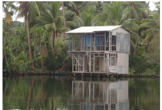
Photo 10. House abandoned due to rising lake level
