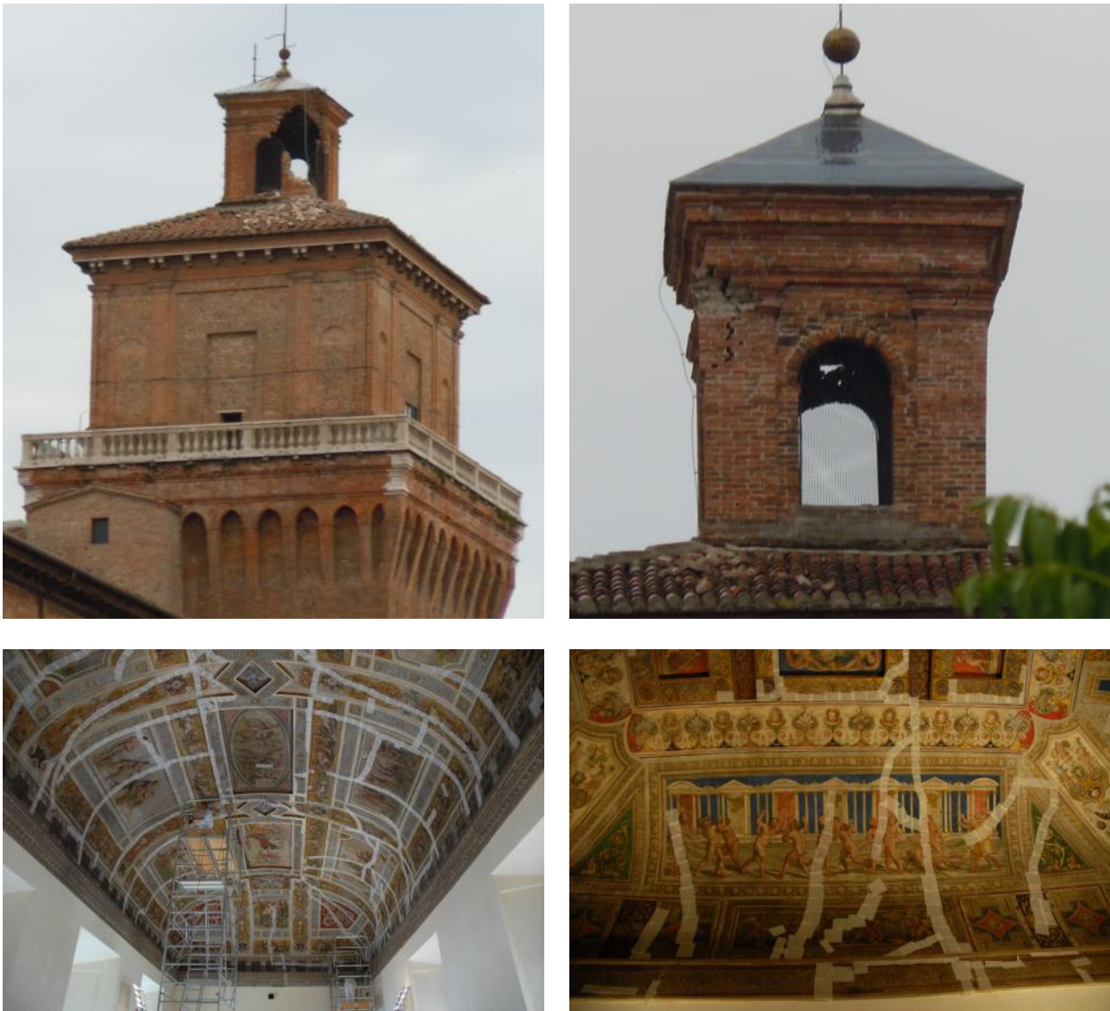
Figure 11 - The two damaged lantern turrets of the Estense Castle of Ferrara (above) and the emergency works to fix the detached frescos (below)
