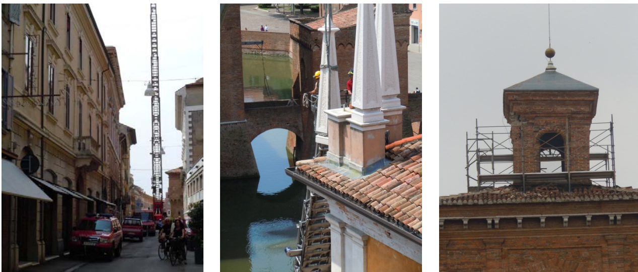
Figure 15 - Initial emergency works to stabilize or remove elements at risk of collapse
