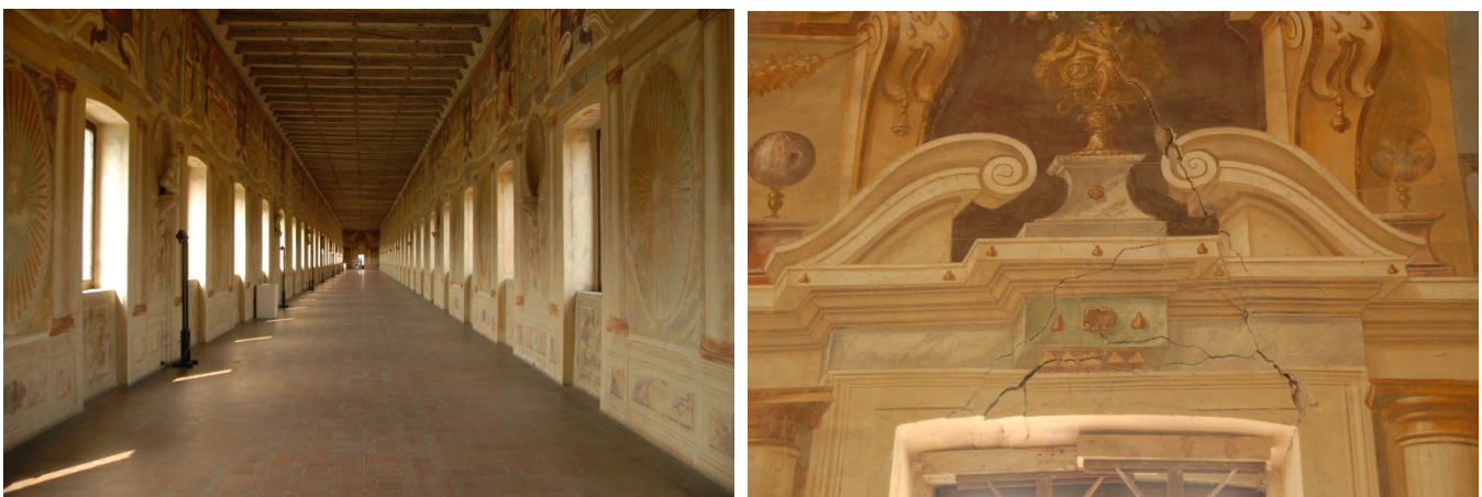
Figure 18 – Sabbioneta, Galleria degli Antichi. General view (left) and cracks over a window of the last bay (right).
