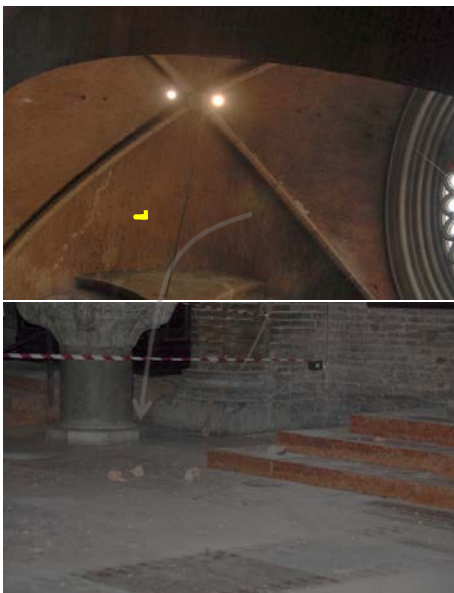
Figure 9 - Bricks collapsed from the vault at the main entrance.
