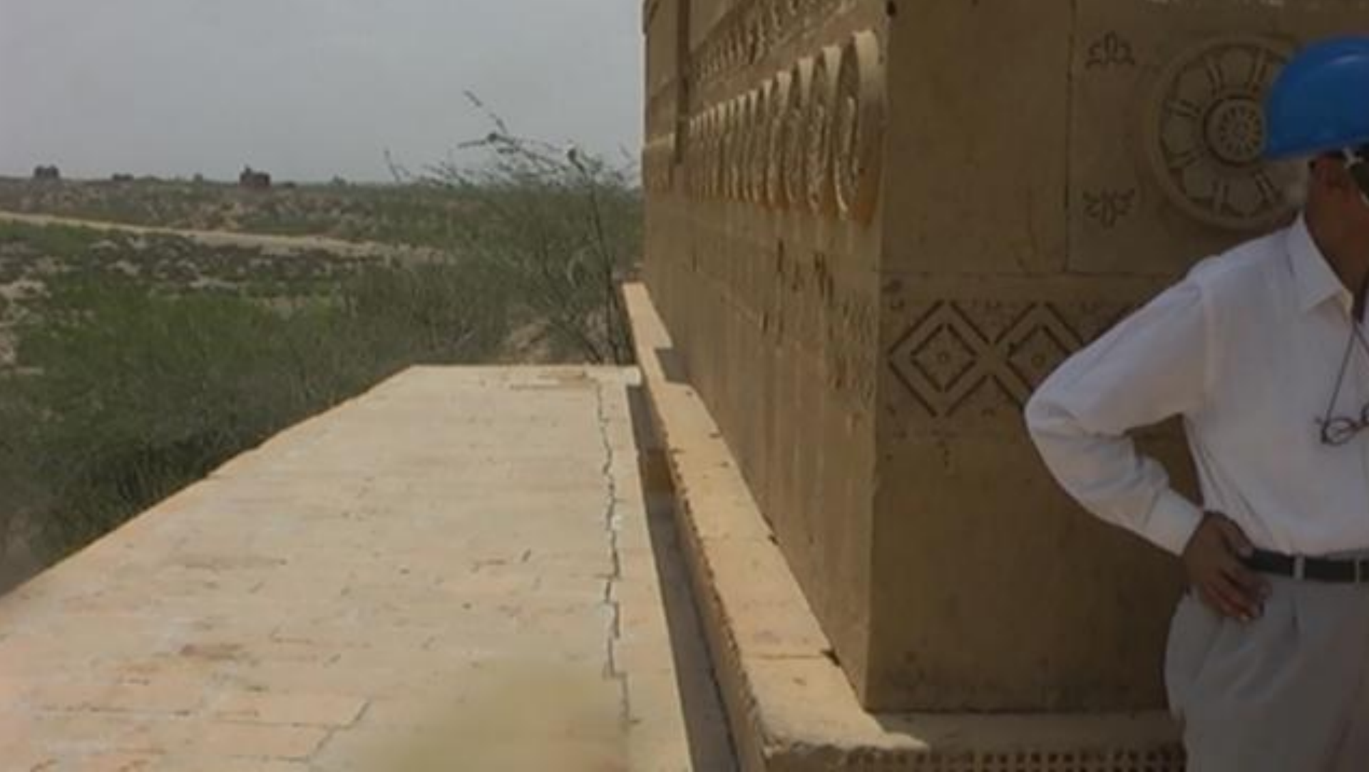
120510 separating cracks of consolidation platform, Jam Nizam du Din
