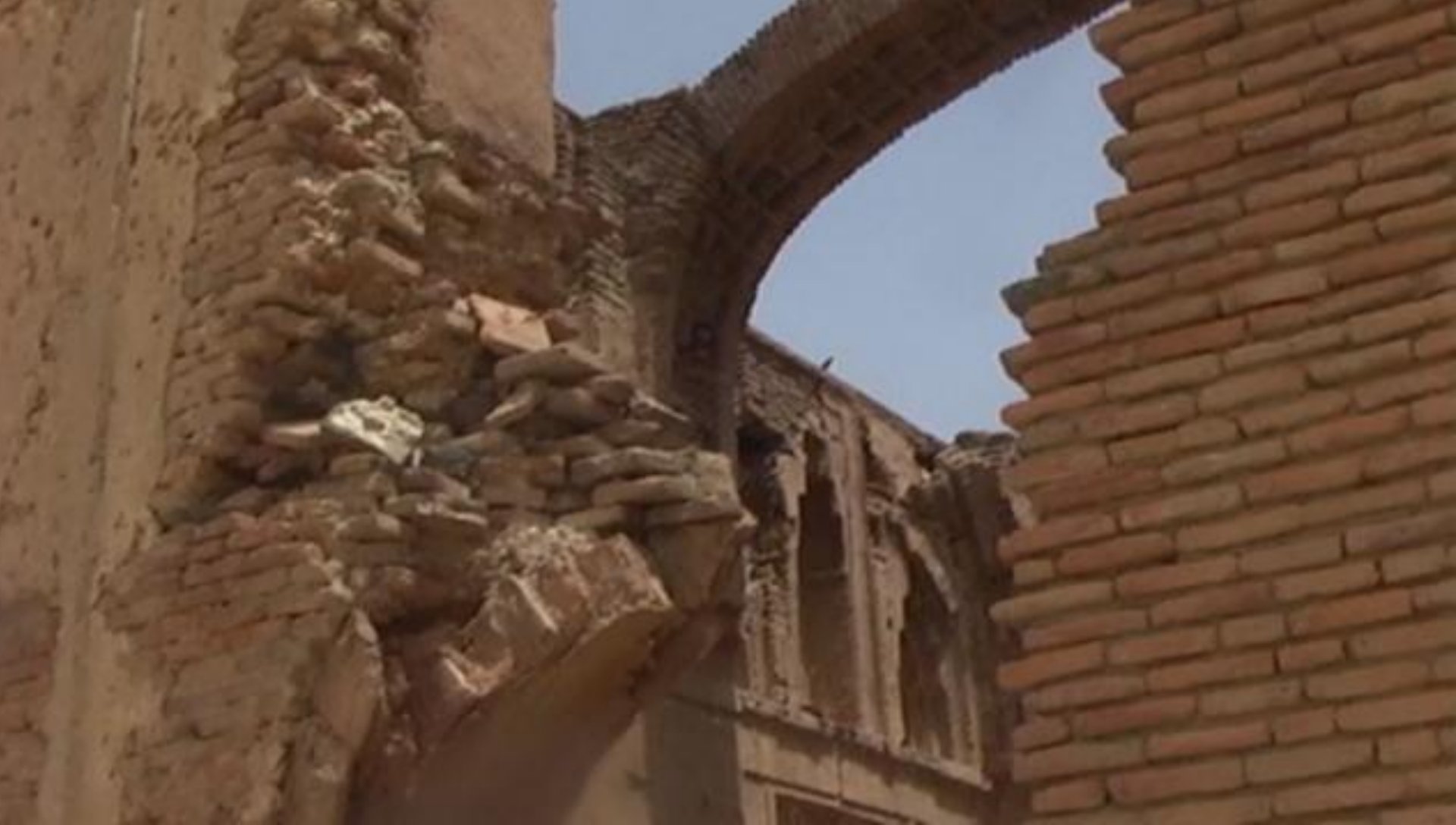
120510 Structural deterioration mosque near Jam Nizamuddin
