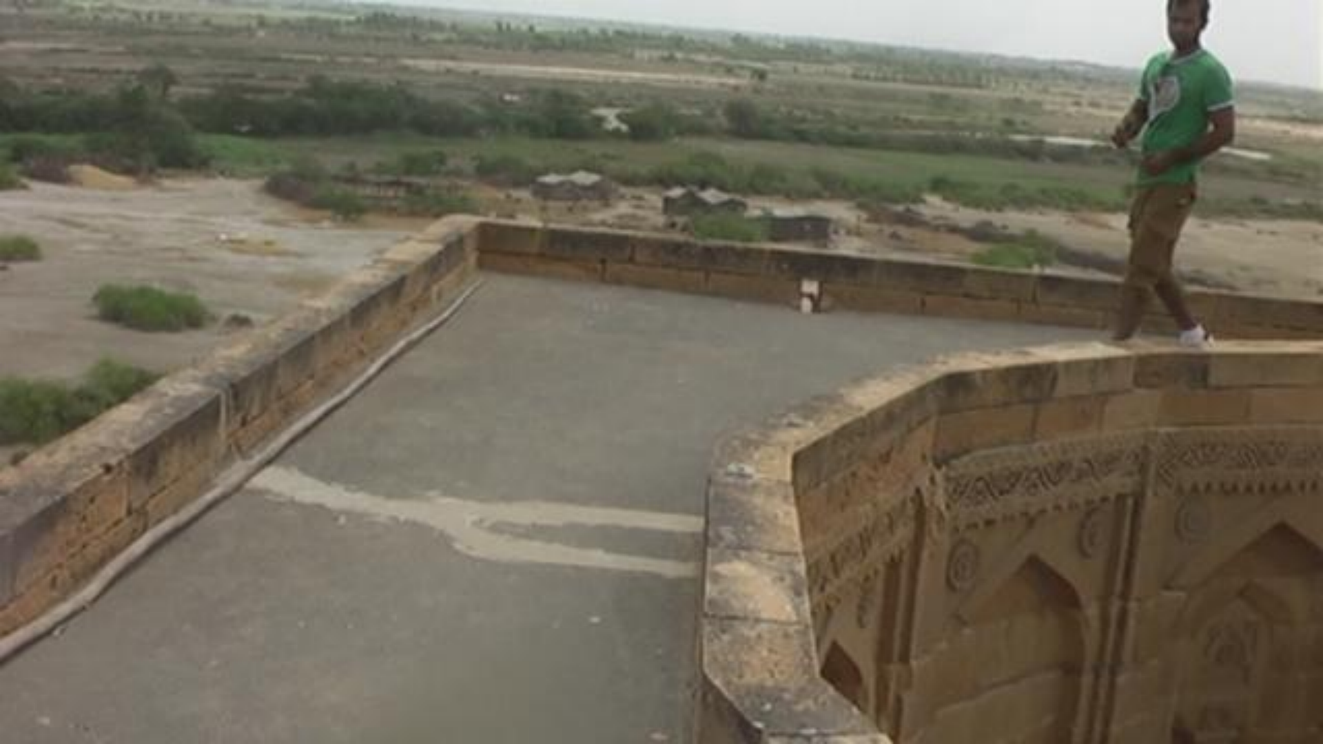
120510 Roof cracks in the Jam Nizamuddin tomb
