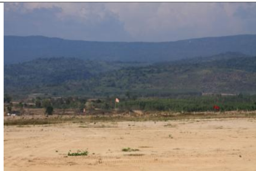
Figure V.4: Construction site of Huay Samong Dam showing flags that indicate the location of the dam ridge
