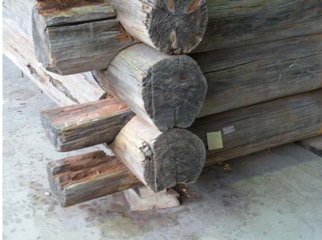
Figure 7 – Typically deteriorated logs from the 7 th tier.
