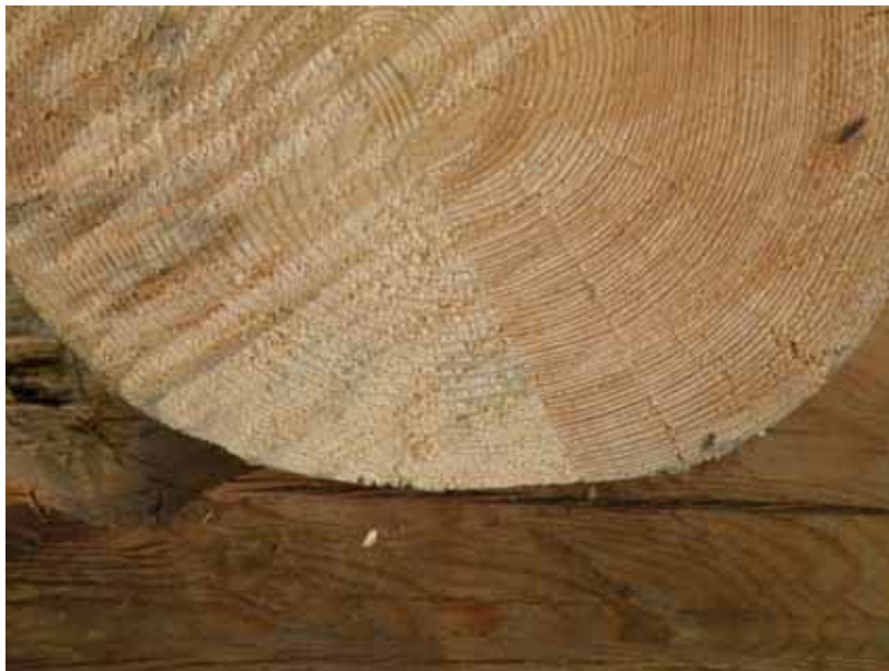
Figure 4 – The best repair is a straight line joint with matching position and size of annular rings. Wood density and moisture content of repairs should match the historic material. This is quite a good match but the annular rings show a significant difference in the density of the two pieces of wood. They will expand and contract differently and should be allowed to do so.
