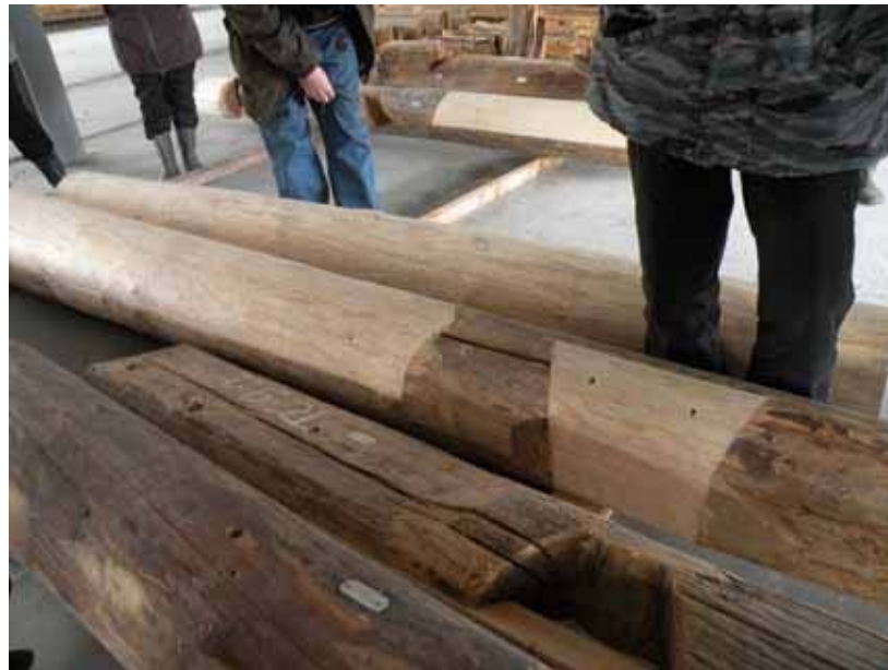
Figure 6 – Multiple repairs in a single log are visually disruptive and non-traditional logwork. Although well made, these joints will have a negative impact on the aesthetic and design character of the building, especially if a single wall has many logs repaired like this.
