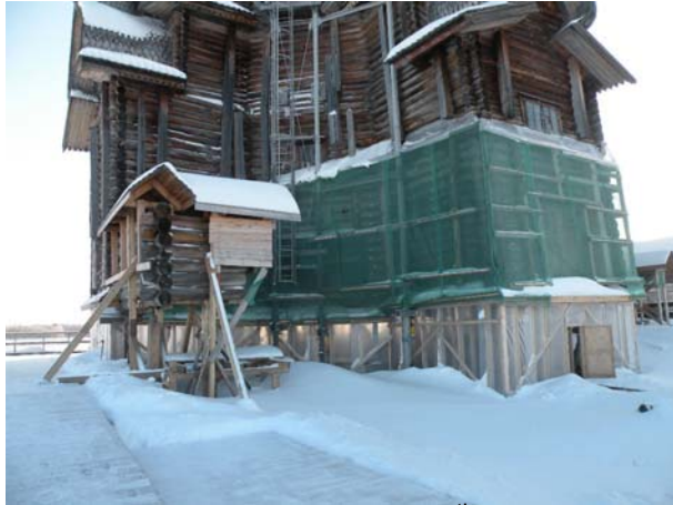
Figure 1 – Church of the Transfiguration with the 7 th tier of logs and the Refectory removed.
