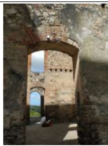
Sans Souci - monitoring the fissure of the arch by a strain gauge connected with a data logger.
