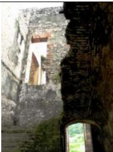
Sans Souci - fissures at the top of the walls may affect the stability of the building.
