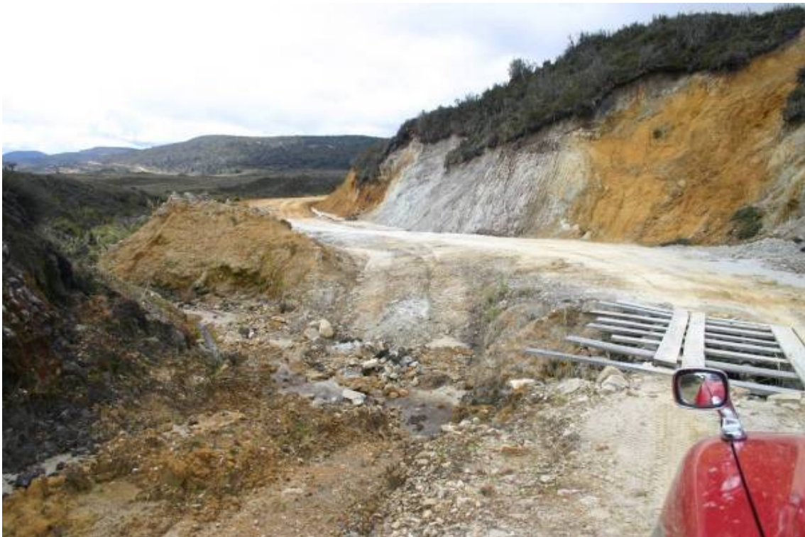
Photo 15: Temporary bridging and extensive erosion on Habema-Nduga-Kenyem road.
