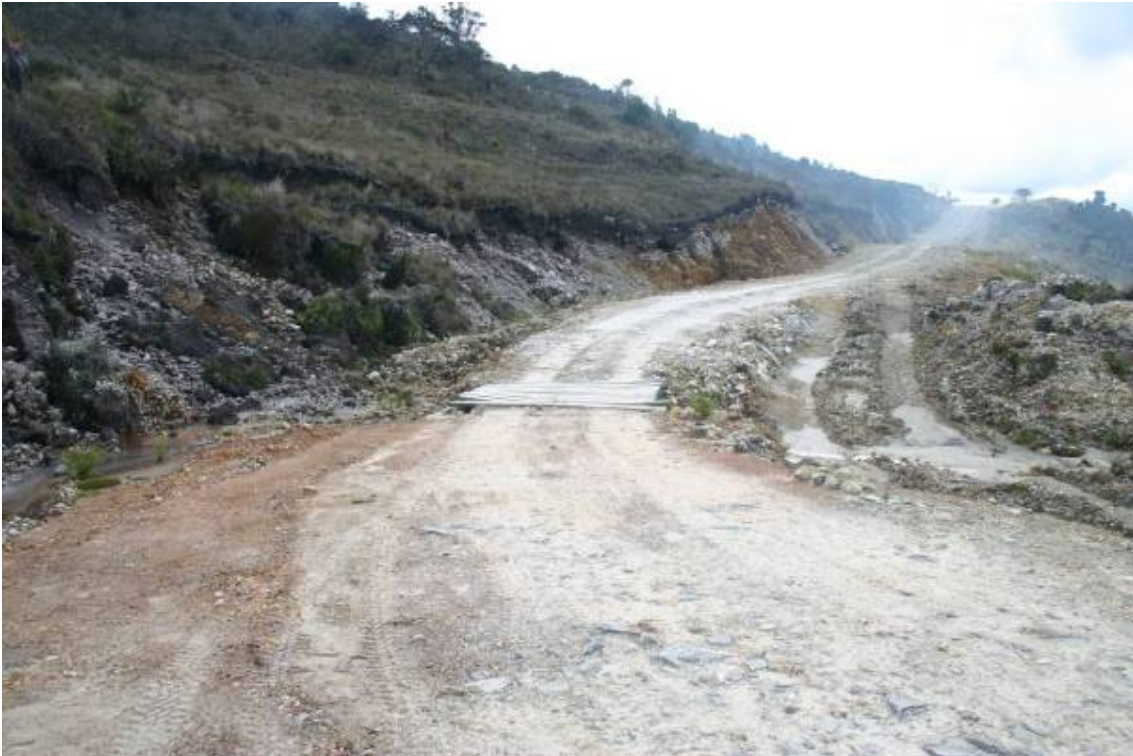
Photo 6: Batter collapse, erosion and track diversion, Lake Habema road.
