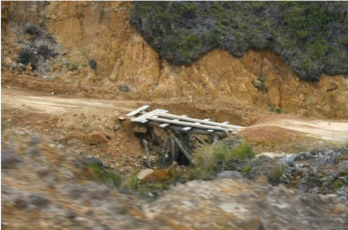
Photo 16: Hazardous bridging and extensive erosion on Habema-Nduga-Kenyem road.
