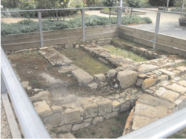
Figure 32 This image shows the same view today. Note vegetation encroachment and mortar deterioration both due to excessive rainwater.
