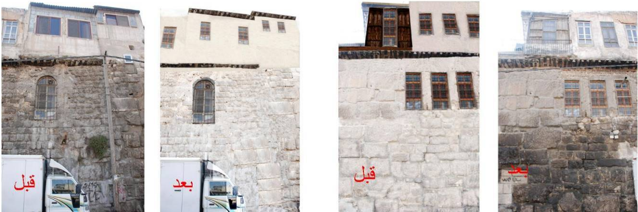
The type of interventions being studied for the restoration of the City Walls (source: Governorate of Damascus - Directorate of Old Damascus)
