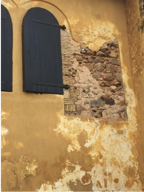
Fig. 15 Problems with failing lime plaster
