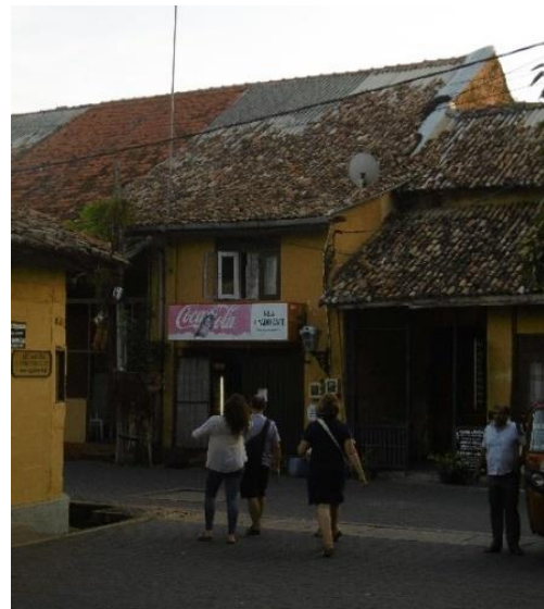
Fig. 12 Tiles slipped on an asbestos cement roof
