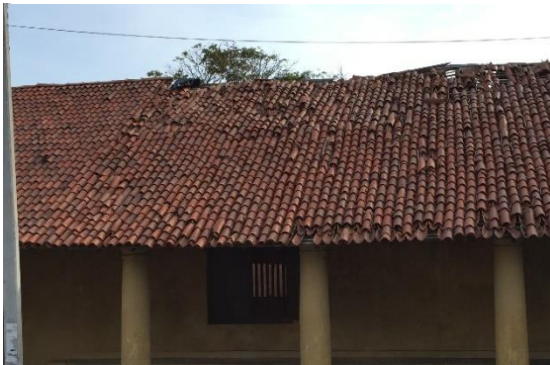
Fig. 18 A derelict property with a roof on the point of collapse
