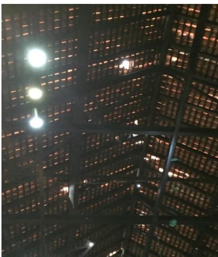
Fig. 13 Daylight showing through the recently retiled roof of the National Maritime Museum
