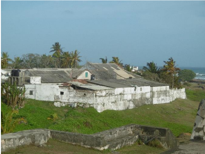
Fig. 9 Buildings currently used by the military and in very poor condition
