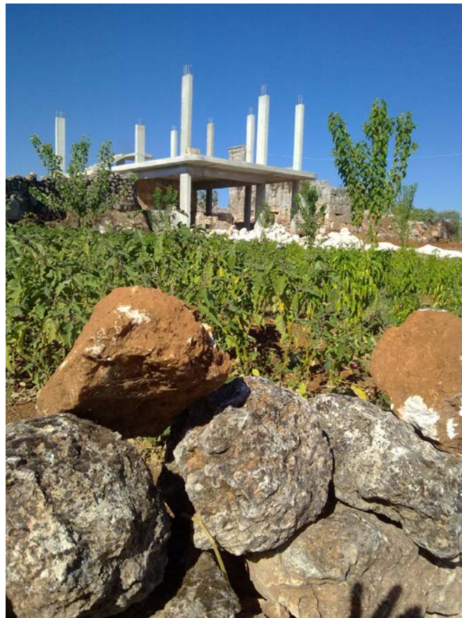
Illegal Buildings at Btressa, Zawia Mountain, Idlib Countryside - © DGAM 2014
