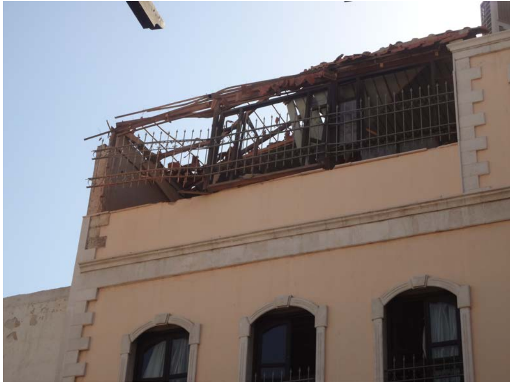
Minor damage to Saada school in al Qanawat historical districts © DGAM 2014
