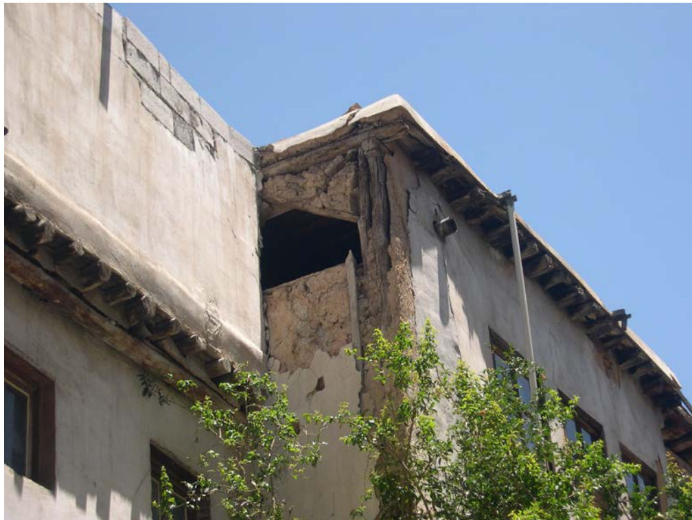
Minor damage to estate n 174 in al Jura districts © DGAM 2014
