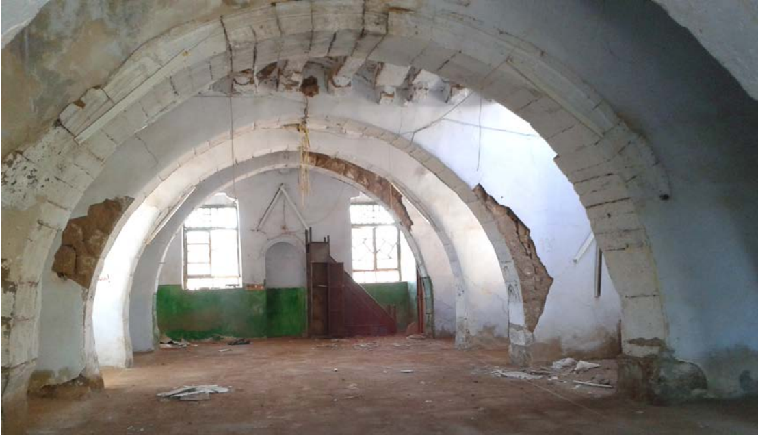
Minor damage to Fatima mosque in Bosra © DGAM 2014
