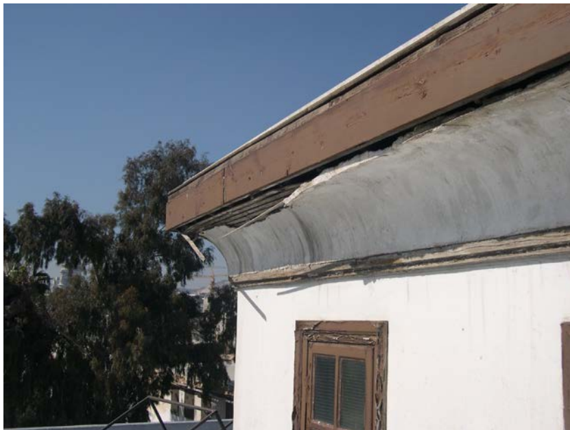
Minor damage to Jukmaqjeh madrasa (The Arab Calligraphy museum) (Estate N468) © DGAM 2014
