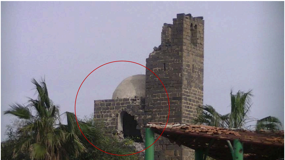
Few stones collapsed in the façade, Abou al Feda mosque, Bosra © DGAM 2014
