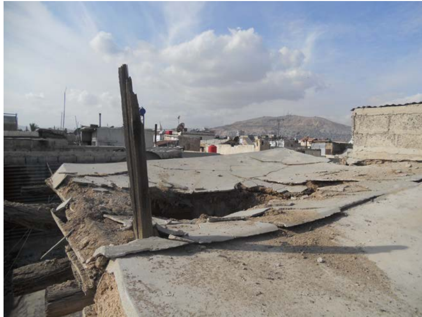
Minor damage to the roof of Beit Al Qwatly in Mezanet Al-Shahem (Estate n468) © DGAM 2014
