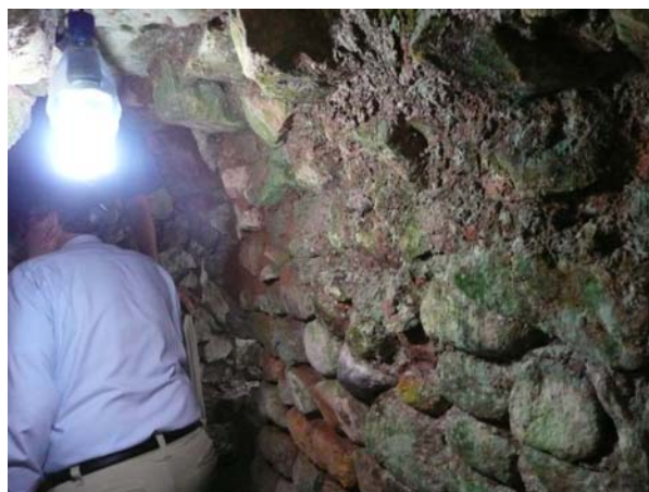
Image 9. Greenish mould on the tunnel surface
