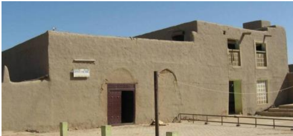
View of the main facade of the Youth House before restoration November 2009
