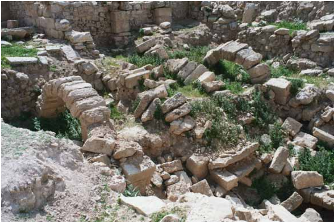
Fig. 8 – ancient structures at the risk of collapse
