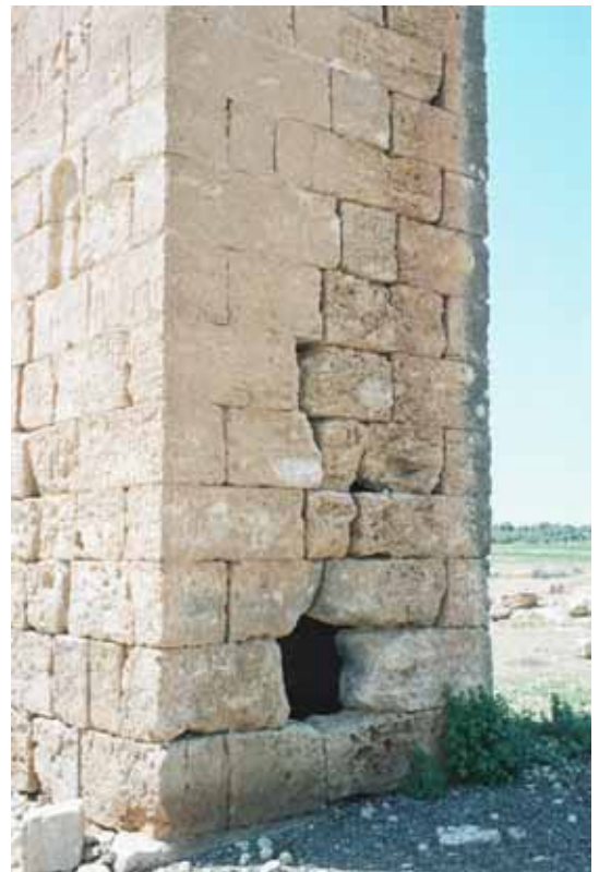
Fig. 26 – structural and erosion damage on the Stylite tower
